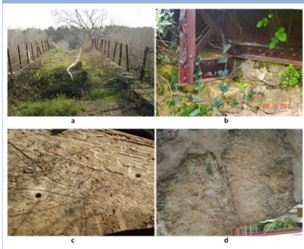
Figure 3: Previous damage status. a) pavement; b) steel structure and adjacent masonry; c) walls; d) ashlar (Conde-Salazar, 2007).
