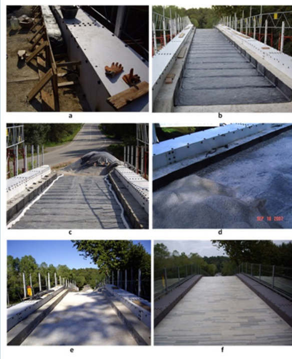
Figure 7: New board construction; a) longitudinal concrete walls; b) placement of waterproofing asphalt sheet. c) two longitudinal drainage pipes; d) two fine gravel layers over asphalt sheet; e) mass concrete; f) stones. (Conde-Salazar, 2007).
