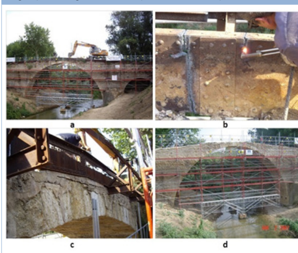
Figure 4: Pavement and metal railing removal (July-August 2007) a) rubble extraction from pavement; b) metal structure removal; c) bridge at its final stage. d) final bridge after removal (Conde-Salazar, 2007).
